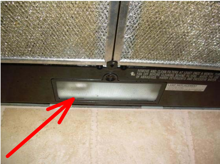
The light for the microwave that is for the stove cooking area doesn't work. Recommend replacement of the stove top light bulb.
