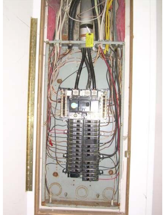
200 amp main electric panel with copper wiring and circuit breaker protection. The panel was in good condition at the time of the inspection.
