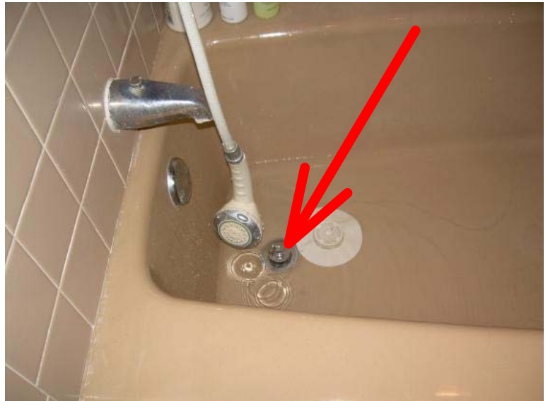
The master bath tub drains very slowly. Recommend cleaning of the drain.
