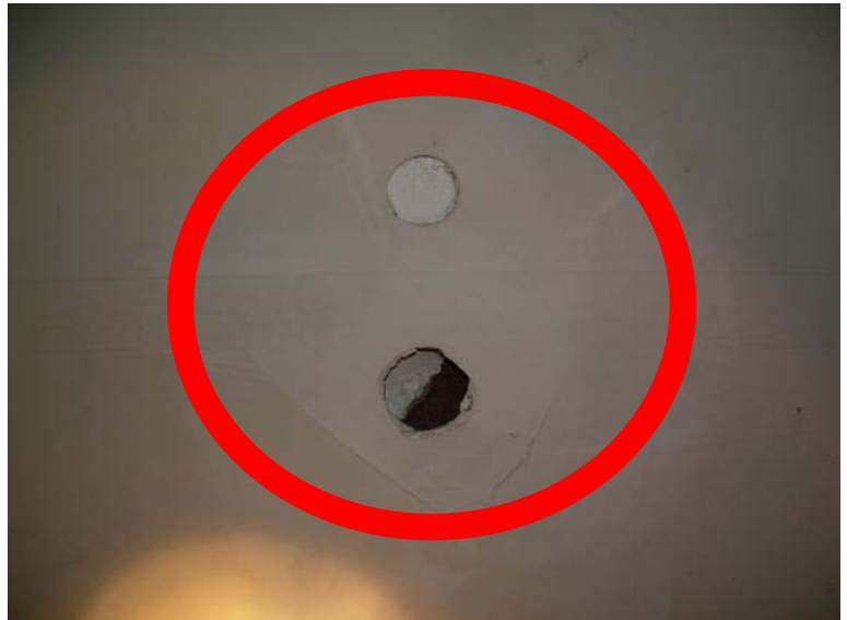
There are several holes in the walls of the garage. Recommend repairs be made to prevent breach of firewall protection.
