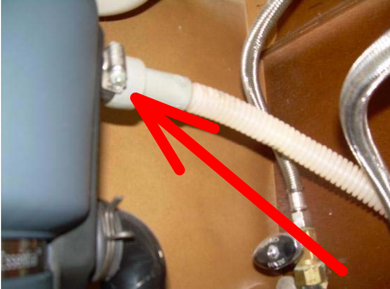
The dishwasher drain is improperly connected to the garbage disposal. This is an area for cross contaminating the water. Recommend having a qualified plumber install the dishwasher drain to the other side of the kitchen sink.
