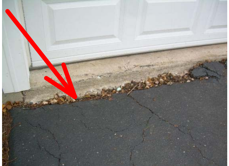
The driveway has settlement near the garage door with signs of previous repairs. Recommend repair or replacement of the driveway.
