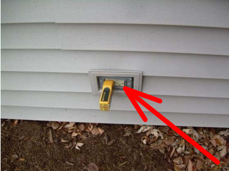
The GFCI outlet at the side of the garage is loose from the wall and is missing a weatherproof cover. Recommend repair or replacement of the outlet by a license electrician.
