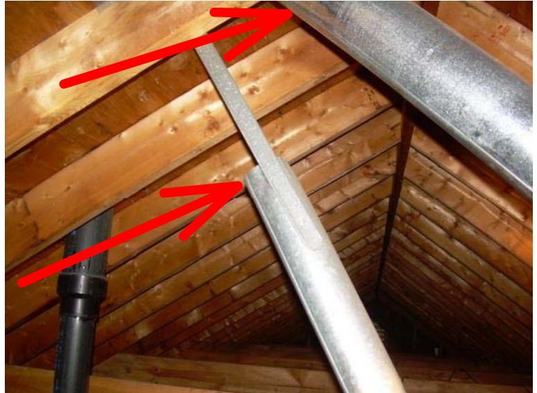
The bathroom vent fans improperly terminate inside the attic area and could cause excessive moisture to build up inside the attic. Recommend having a qualified contractor extend vents to the exterior of the home.
