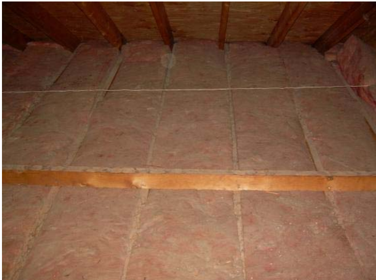
Recommend additional insulation be added to the main attic for better efficiency. There is only 6 inches of insulation present.
