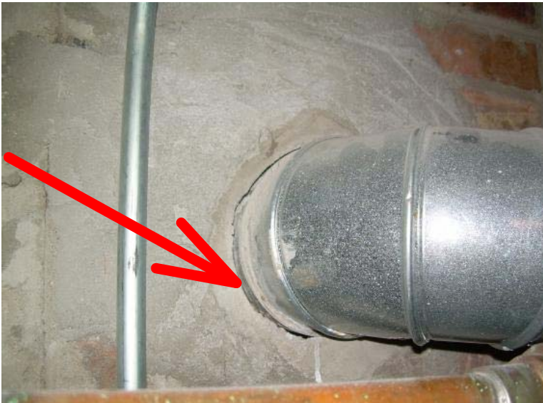
Where the furnace flue piping enters the masonry chimney there is a large gap between the piping and the brick. Recommend sealing with appropriate sealer by a qualified heating contractor.
