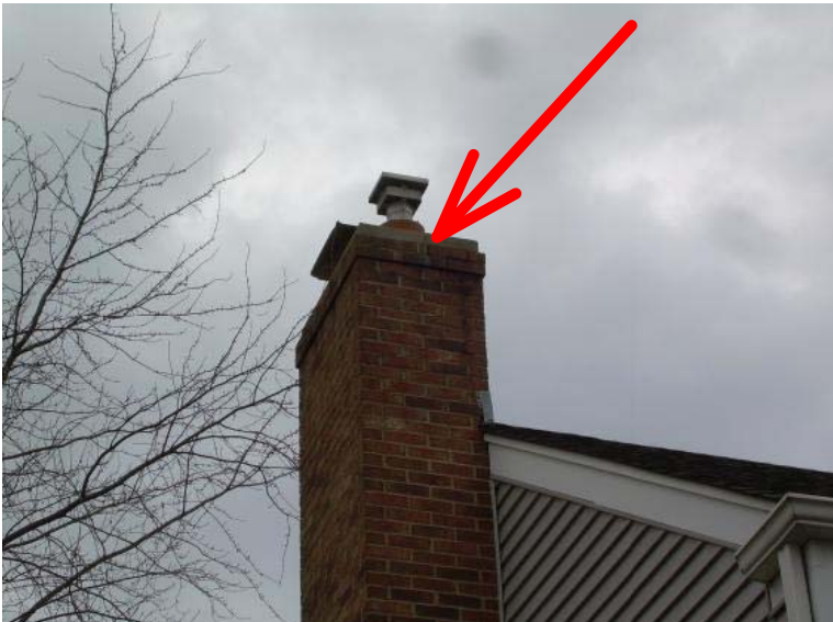
The chimney cap is cracked and in need of repair to help prevent moisture penetration.
