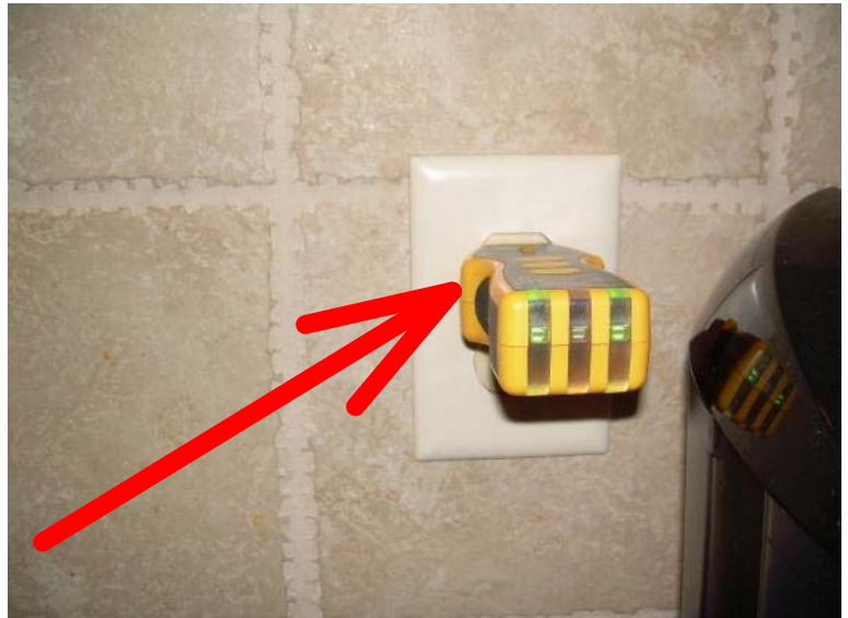
The kitchen wall outlets are not GFCI protected Recommend adding GFCI outlets to the kitchen for safety near water.
