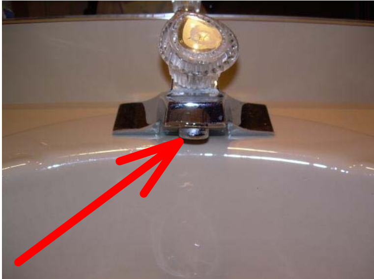
The left faucet in the upper hall bathroom has a leaking filter screen and is partially clogged. Recommend replacement of the filter screen.
